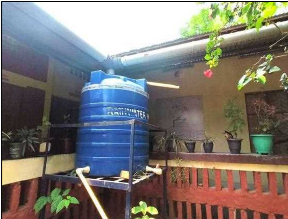
ROOFTOP RAIN WATER HARVESTING SYSTEM
